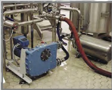
■ Brewing - Pumping Kieselguhr
