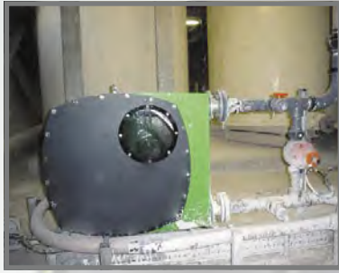
■ Water treatment - Lime mixing & recirculation
